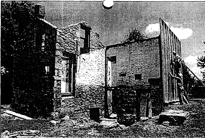
Preparing for its relocation to Hobbs Park, Dan Rockhill and Assoc., encase the house in a wood "box" to minimize damage during the move.
